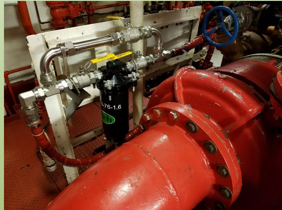
Fitch model FHD20 installed on starboard engine
